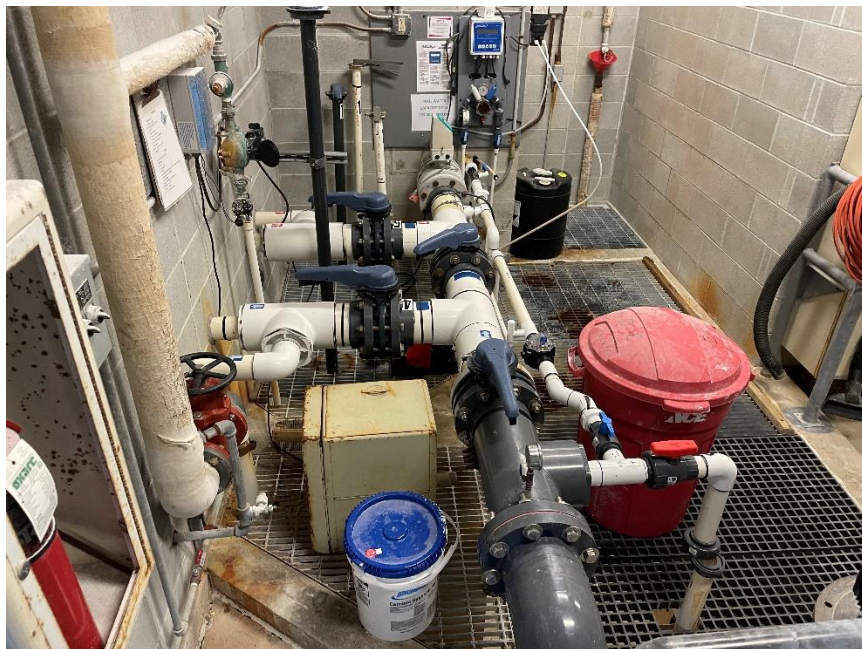
Plate 10 – Corroded Grating Panels
