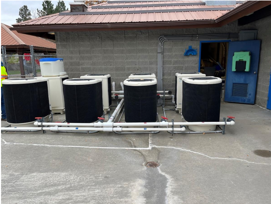
Plate 12 – Pool Heat Pumps
