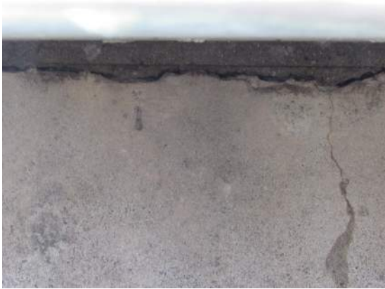
Cracking in the back of gutter
