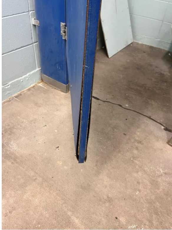
Plate 7 – Stall Door Delamination
