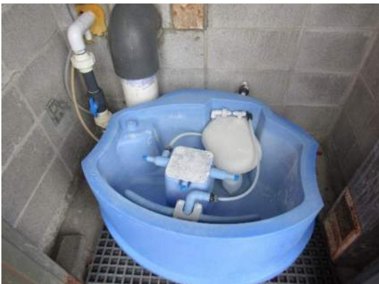
Calcium hypochlorite erosion feeder
