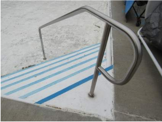
Entry steps with handrail, not ADA compliant
