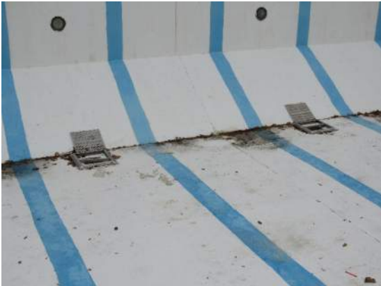
Main drains in diving well
