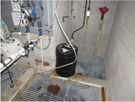
Hydrochloric acid stored in mechanical room
