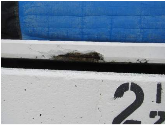
Gutter parapet with chipping and cracking
