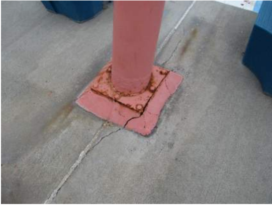
3-meter diving board stand base, severely corroded and cracking
