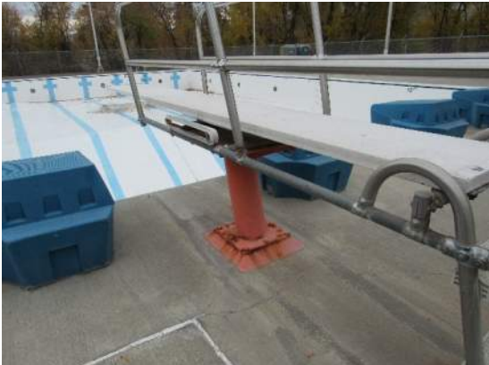
1-meter diving board with severely corroded stand base
